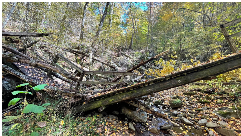
Figure 2. Pictures of the existing bridge looking upstream, damaged in 2019. Picture taken on October 14, 2022.
