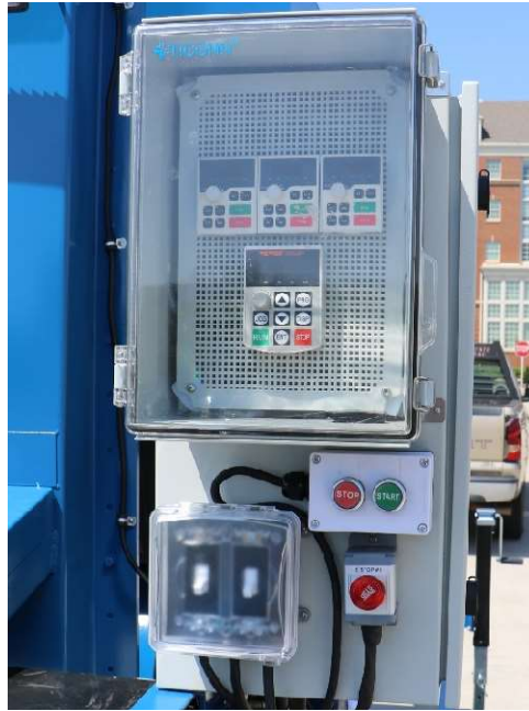
Figure 17: Electrical control panel.
